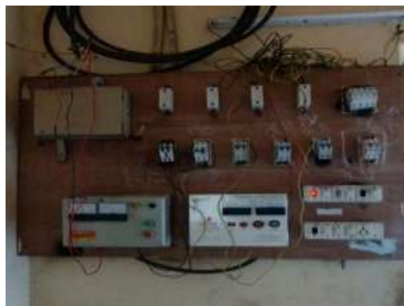
Proper safety precautions should be taken for panel board
